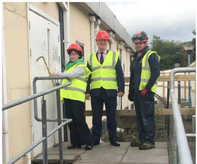
To kick off the removal of the old prefab the honours were given to Clodagh Byron Telephony Manager who was the first staff member to start work in the portakabin and ironically also the last. She was supervised by Ciaran Faughnan Director of Facilities & Estates and Adam Zylan from Hegarty Demolition, Clodagh thoroughly enjoyed the experience!
